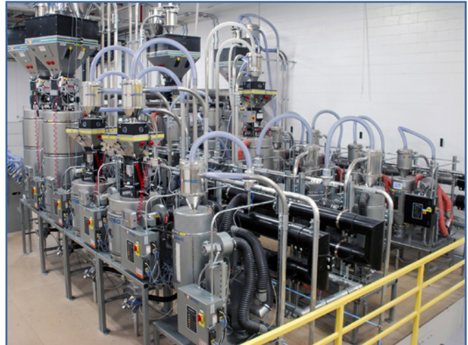
Compact Drying, Blending and Conveying area
